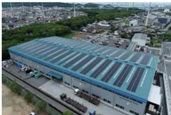
The solar power generation system can produce approximately 600,000 kWh/year, which is sufficient to cover the annual power consumption at the product warehouse and the head office.
