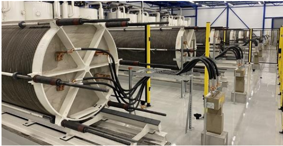
Electrolyzer of hydrogen plant of OVAKO
