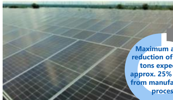
Solar power generation
