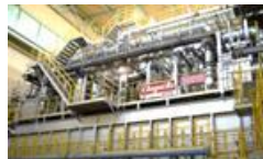
Energy-saving heating furnace that uses regenerative burners
