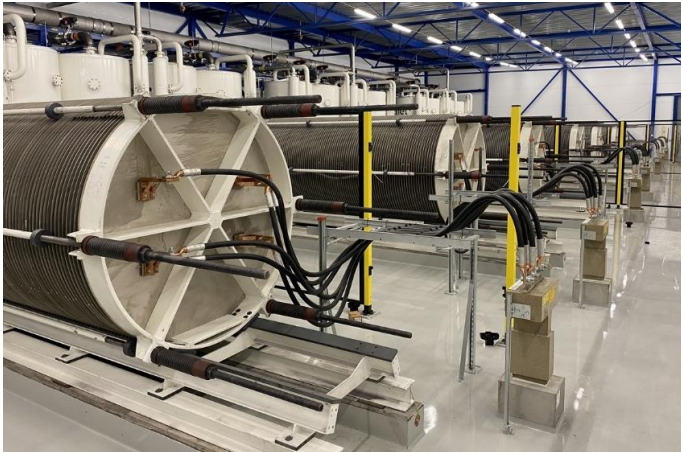
Electrolyzer of hydrogen plant of OVAKO
