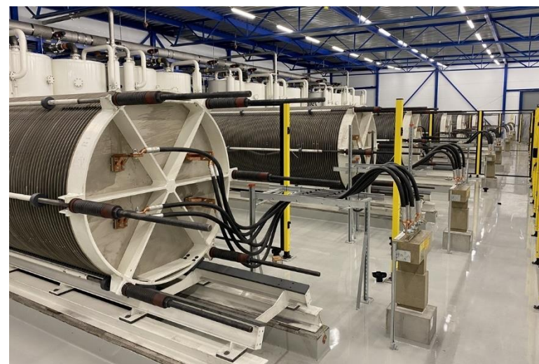
Electrolyzer of Hydrogen plant of OVAKO
