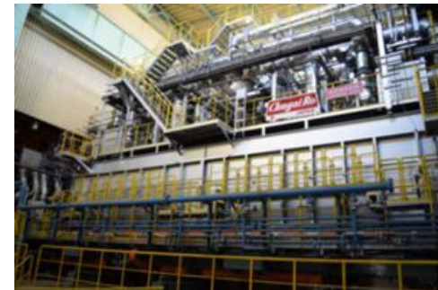
New heating furnace
