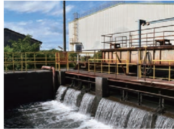
Wastewater treatment facility
