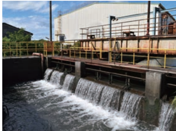
Wastewater treatment facility
